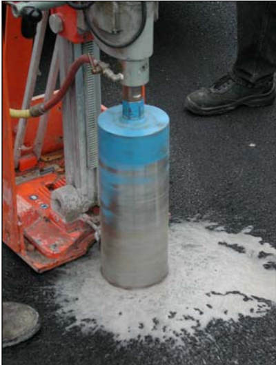
Fig. 12 - Asphalt boring with a Milwaukee Cat. No. 4004/4 machine, equipped with 160 mm diameter borer
