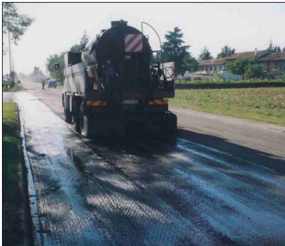
Fig. 8 – Spraying of the tack coat from a tank truck with spraying bar.
