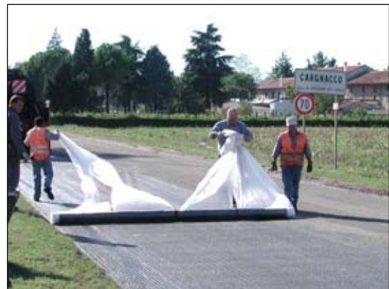
Fig. 7 - Two workers can lay down a whole roll of ARTER® GTS A geogrids, 100 m long, in few minutes
