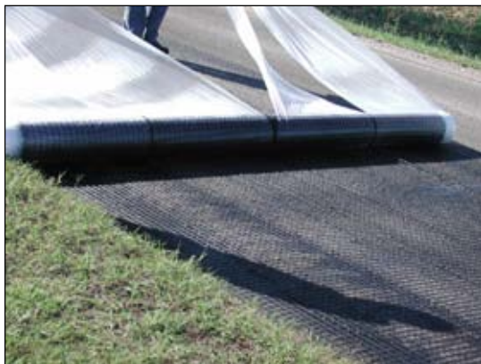
Fig. 6 – By pulling the Polyethylene sheet, the Geogrid unrolls uniformly on the support layer, without creating folds or waves
