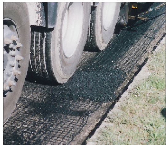
Fig.9 – A small quantity of asphalt on the first metre of Geogrid and along side edges allows to keep the roll in the right position.
